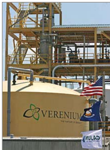
Lake Charles (La.) American Press Verenium's "cellulosic" ethanol pilot plant in Jennings, La., has been designed by the alternative energy company to run on agricultural waste and wood products instead of corn.
